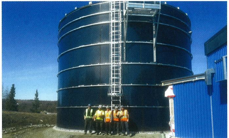
Kuujuaq's tank, which is 11.9 m in diameter by 9.14 m tall, took less than 15 days to erect.
